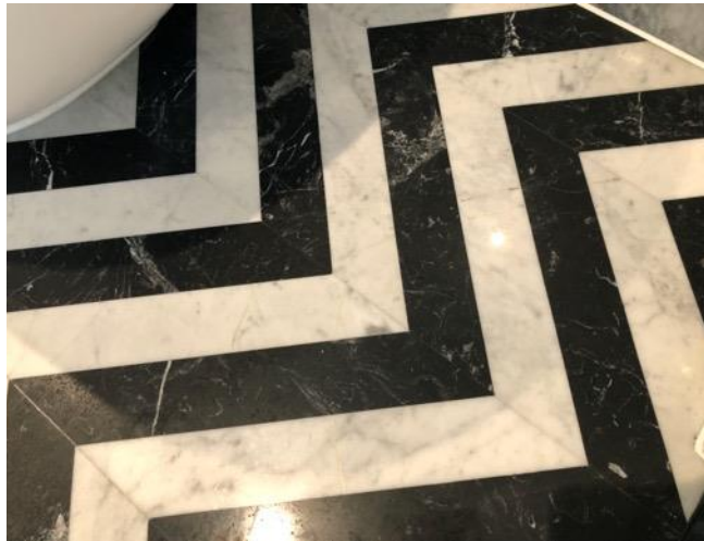
Hairline cracking to floor 2
