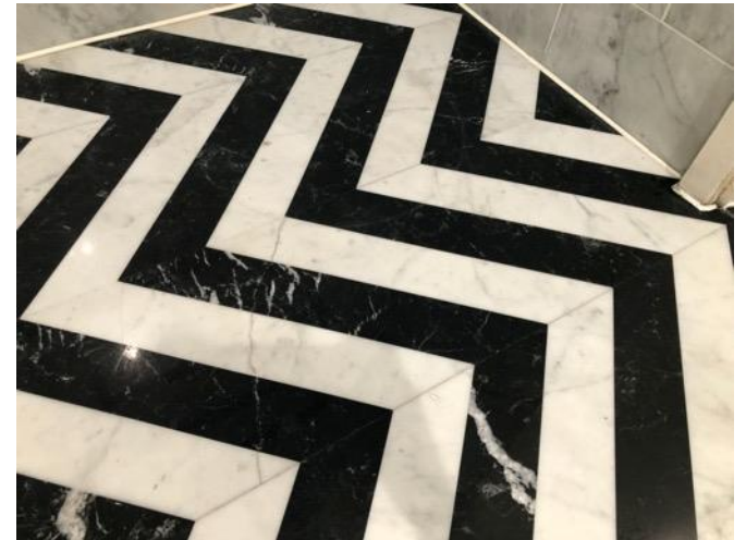
Hairline cracking to floor 5
