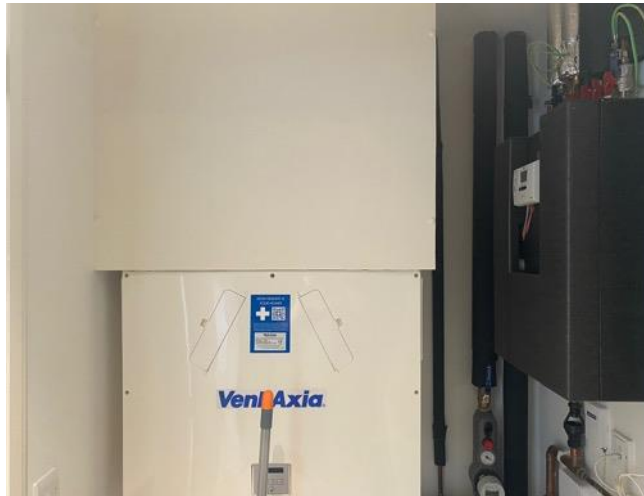
Utility cupboard (angle 2)
