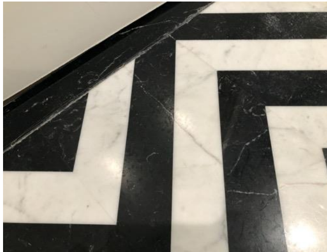
Hairline cracking to floor 4
