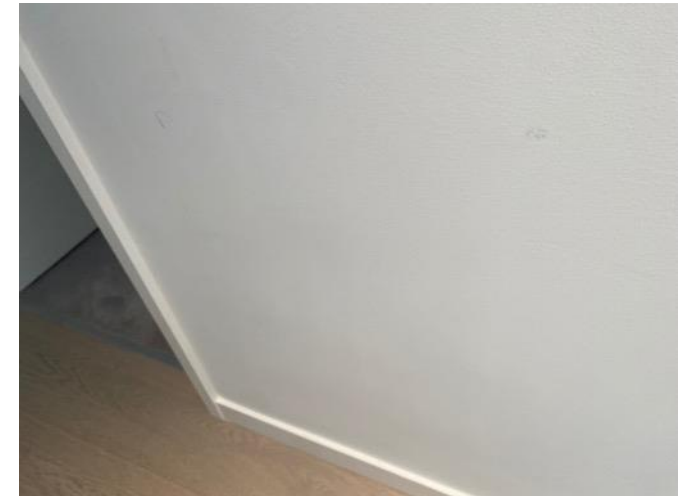
Light scuffs to walls 1
