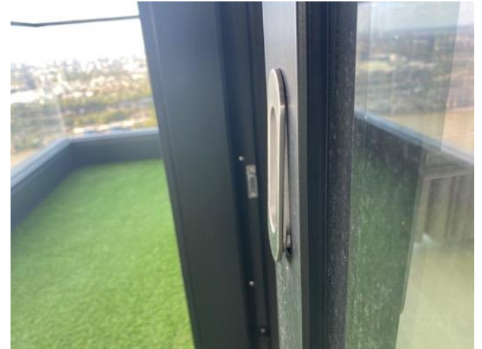
Exterior balcony door handle loose in fittings
