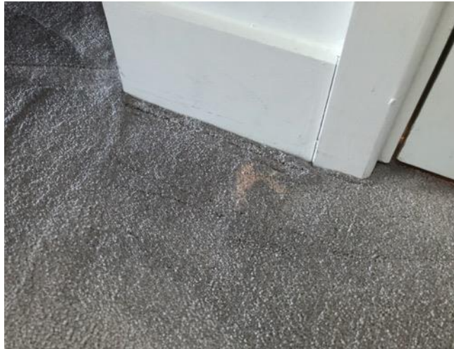
Bleached mark to carpet lhs entry
