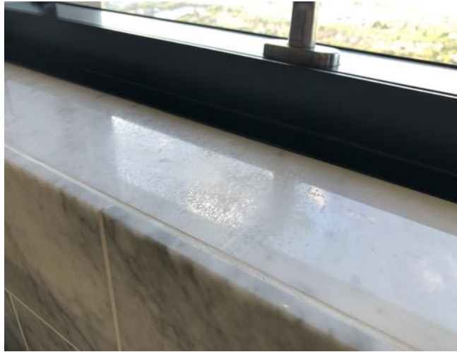
Light limescale marking to window sill
