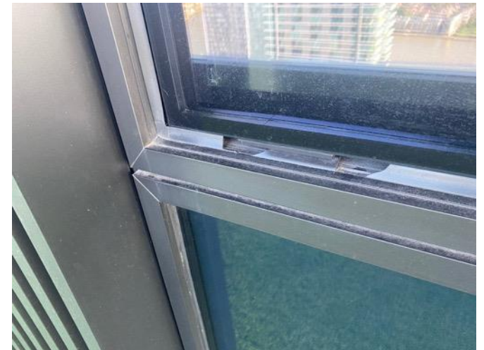
Damage to exterior window frames 1
