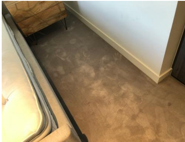
Condition of carpet 6
