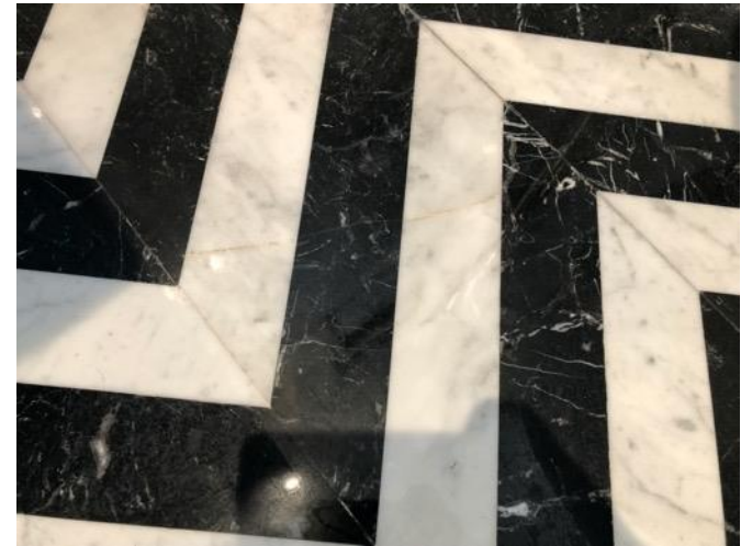
Hairline cracking to floor 3
