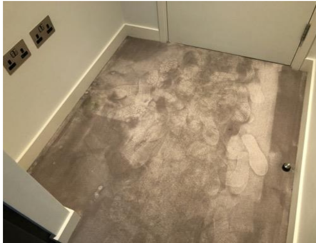
Condition of carpet 8
