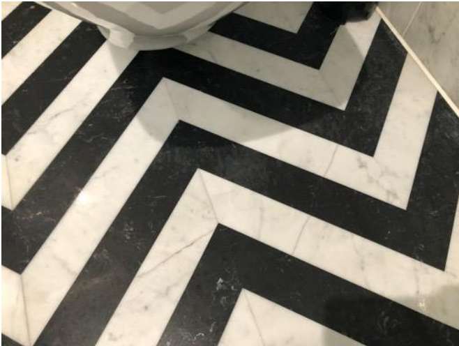
Hairline cracking to floor 1
