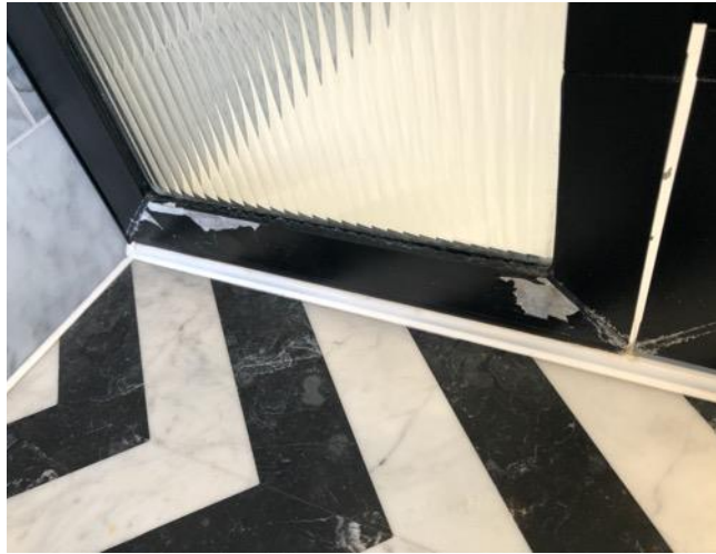
Paint chipping to shower door frame low level
