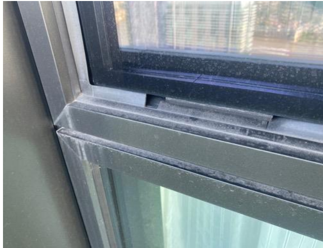
Damage to exterior window frames 3
