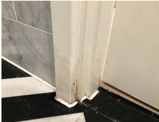
Paint cracking to door frame low level 2
