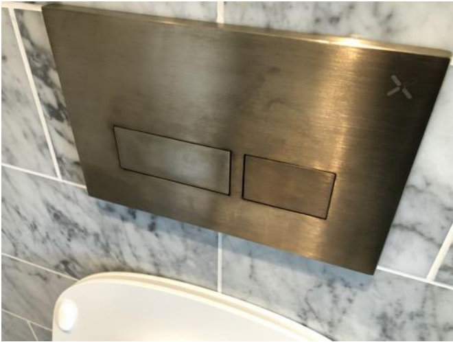
Tarnishing to toilet flusher plate
