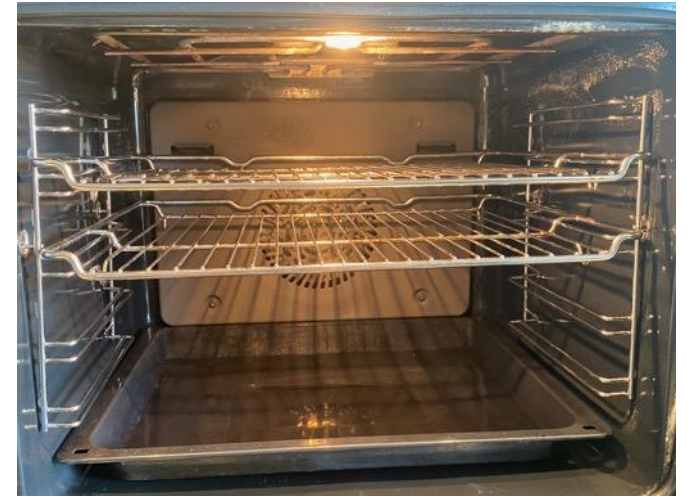
Condition of kitchen oven 2
