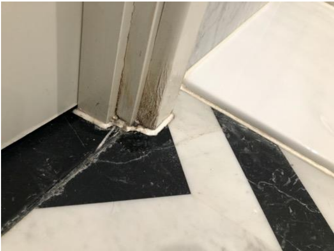
Paint cracking to door frame low level 1
