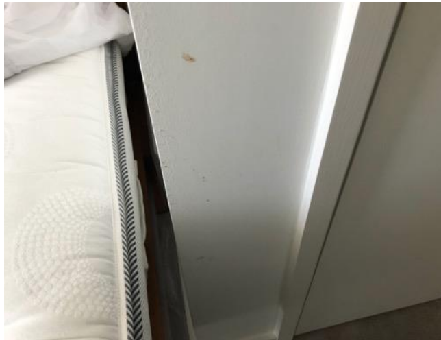
Grubby marks to wall
