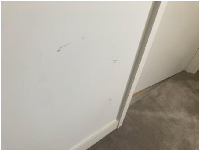
Scuff marks to wall
