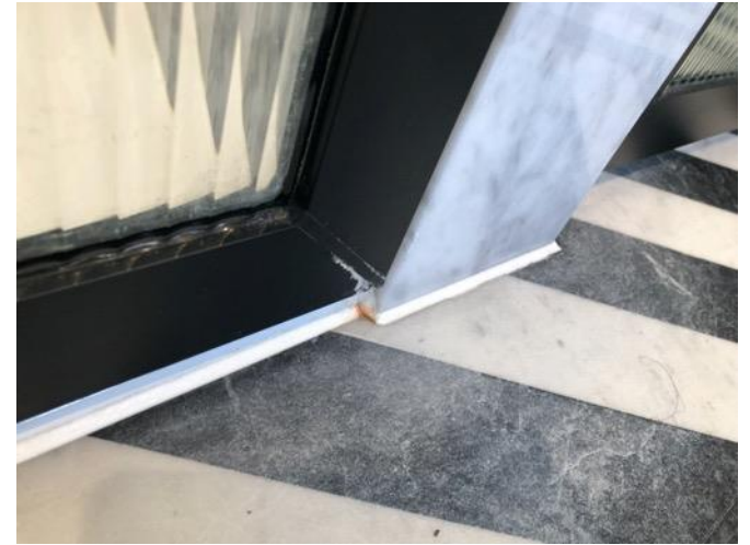
Orange mark to sealant around shower door frame rhs
