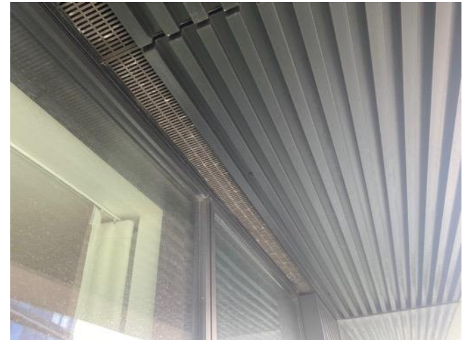
Light staining to overhead vent outlet panels
