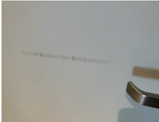
Scratch line to exterior door
