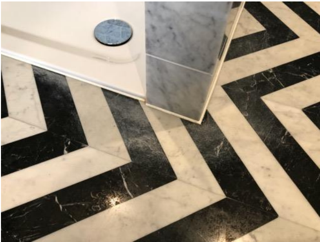
Limescale marking to floor around shower and toilet area
