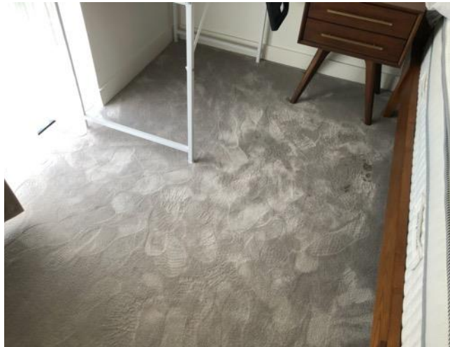
Condition of carpet 3
