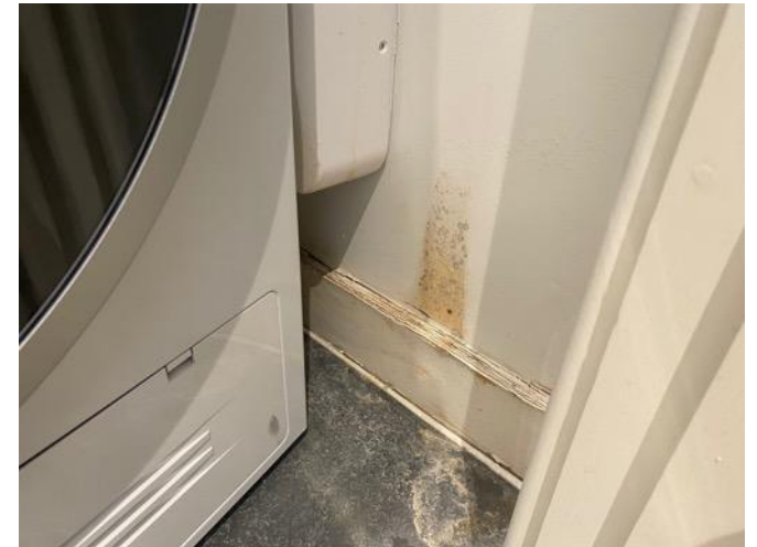
Water damage to utility cupboard wall/skirting/floor
