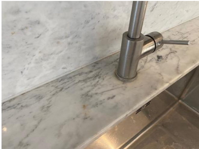
Light discoloured mark to worktop
