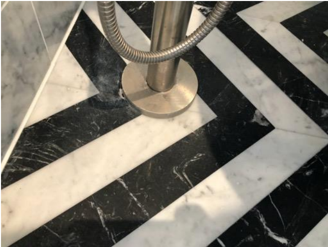
Limescale marking to floor around bath fittings
