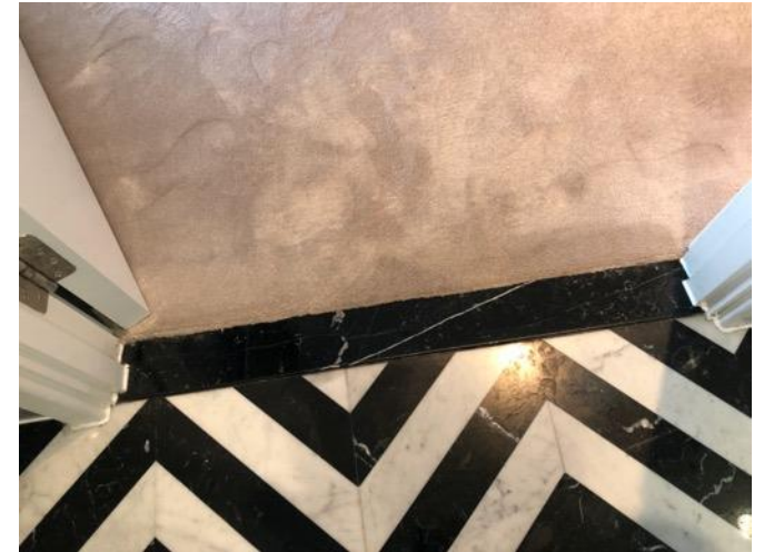
Hairline crack to threshold
