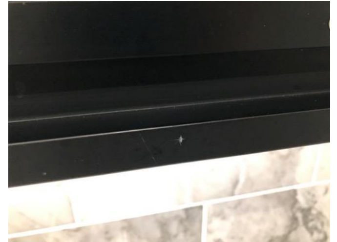
Light marks to interior of cabinet
