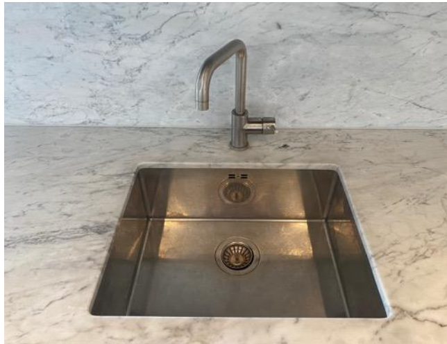
Condition of kitchen sink
