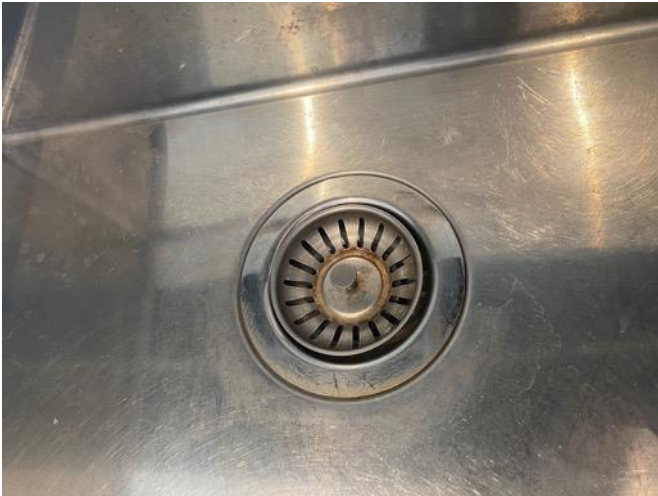
Tarnishing around edge of sink plug
