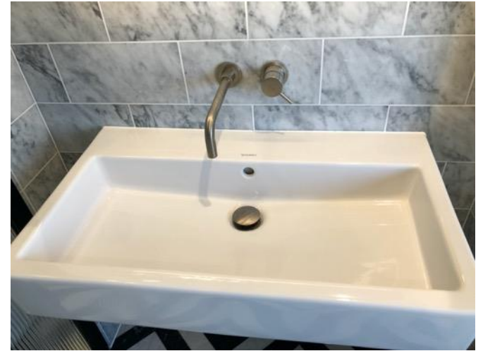
Condition of hand basin
