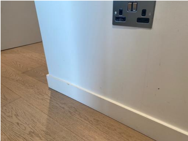
Light scuffs to walls 2
