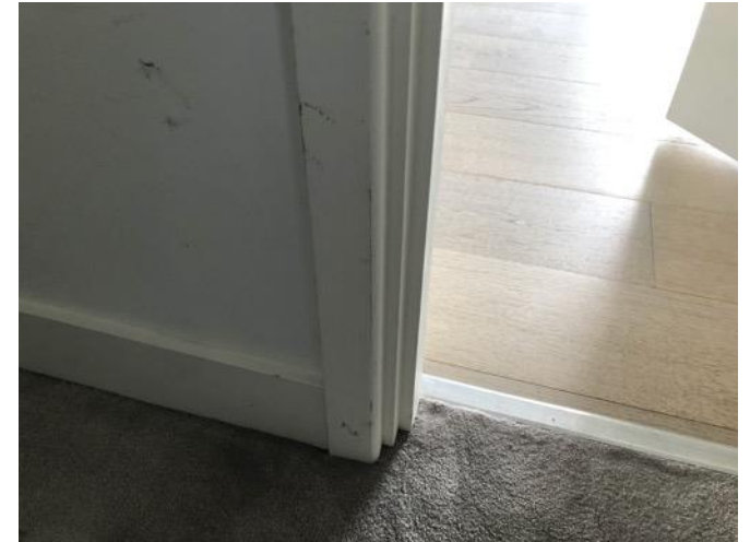
Scuff marks to door frame (to reception)
