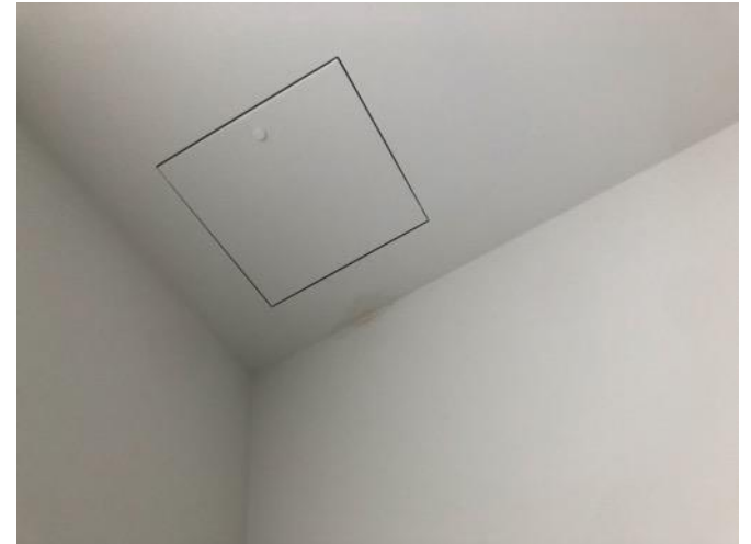
Patchy stain to ceiling/wall join
