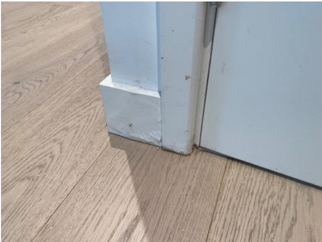
Water damage to skirting 2
