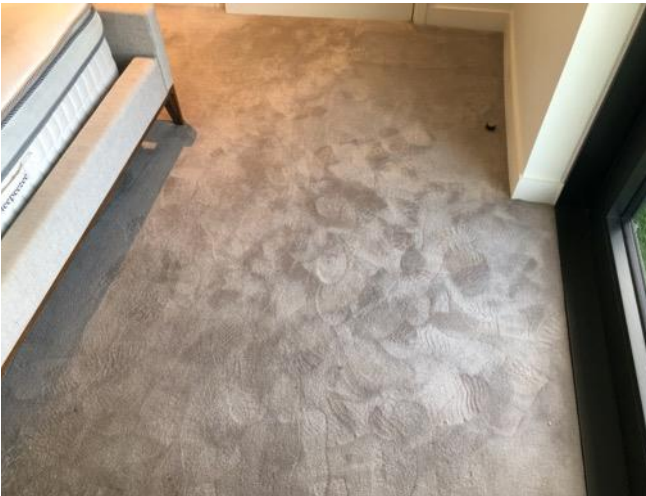
Condition of carpet 1
