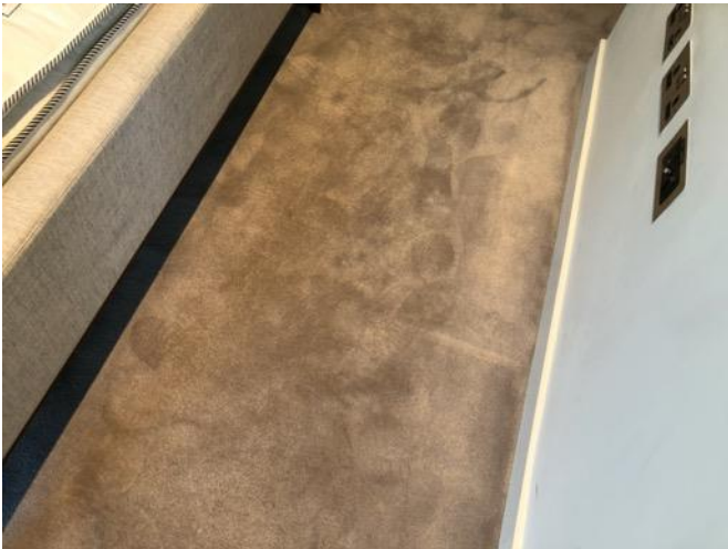
Condition of carpet 4
