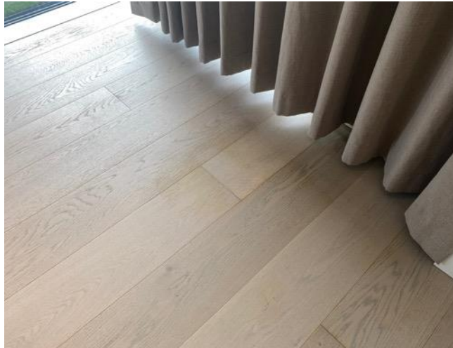
Discolouration to floorboards near balcony door
