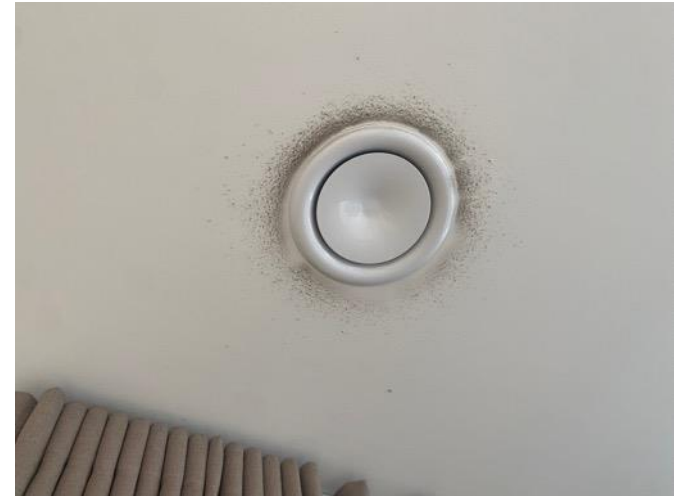
Spotting to ceiling around vent outlet
