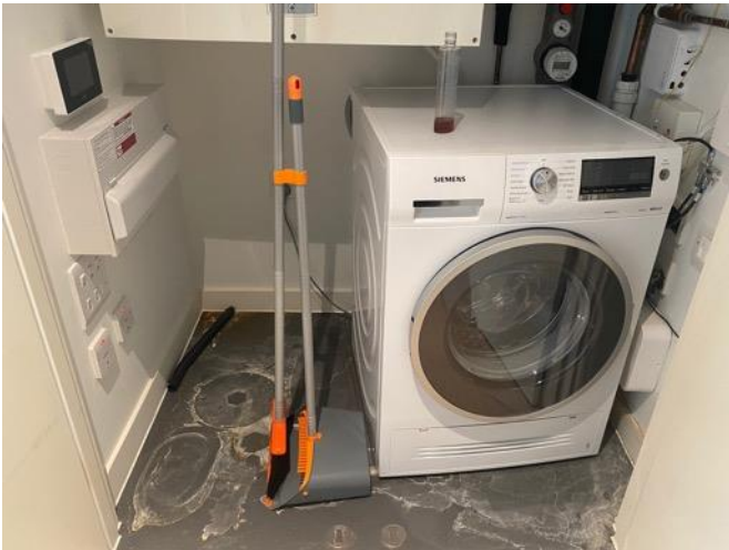
Utility cupboard (angle 1)
