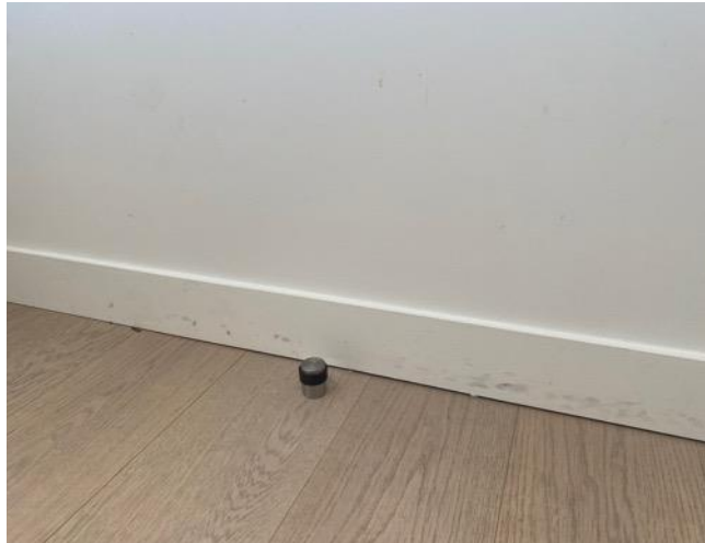
Scuffing to skirting opposite island
