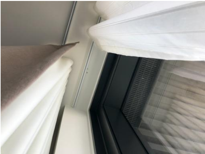
Hole to ceiling behind curtain track
