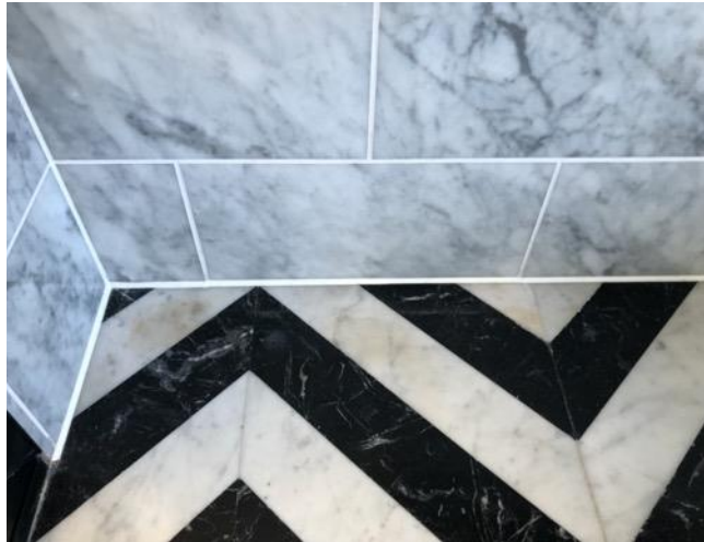
Patchy discolouring to floor below hand basin
