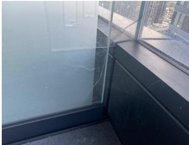
Cracking to far end adjoining glass panel
