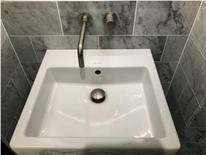
Condition of hand basin
