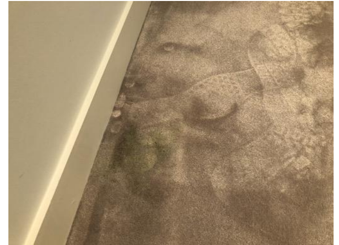
Green staining to carpet rhs upon entry
