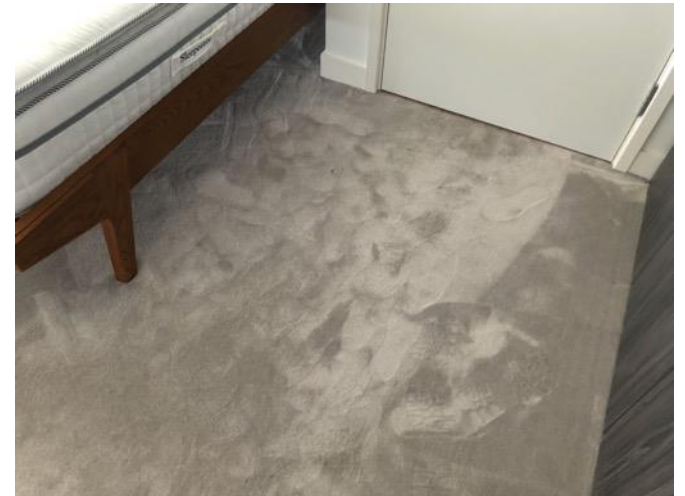
Condition of carpet 1
