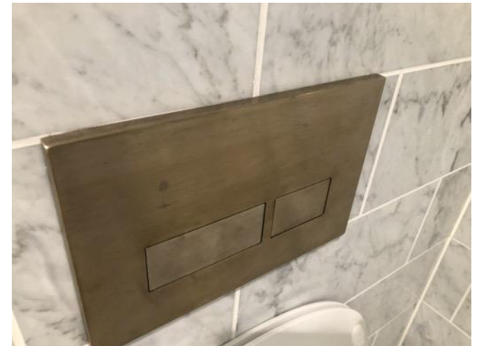
Tarnishing to toilet flusher plate
