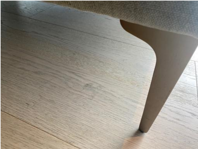
Light scuffs to floor 2
