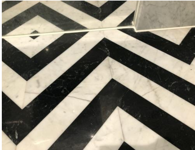
Hairline cracking to floor 2
