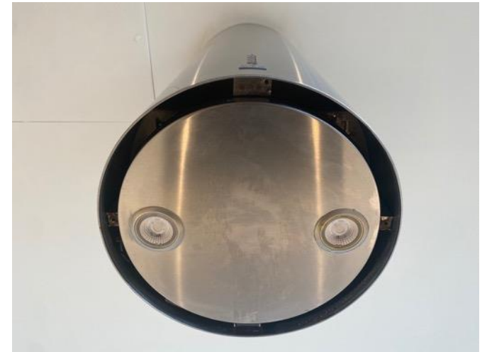
Condition of kitchen extractor unit
