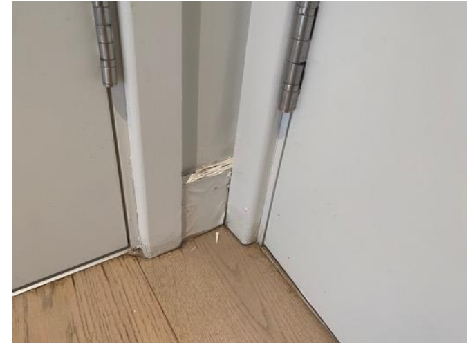
Water damage to skirting 1
