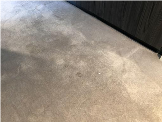
Dark marks to carpet in front of wardrobe rhs
