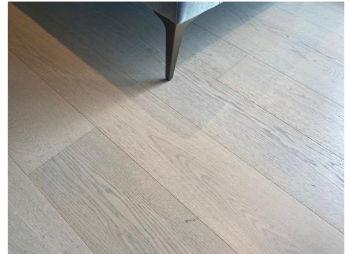
Light scuffs to floor 1
