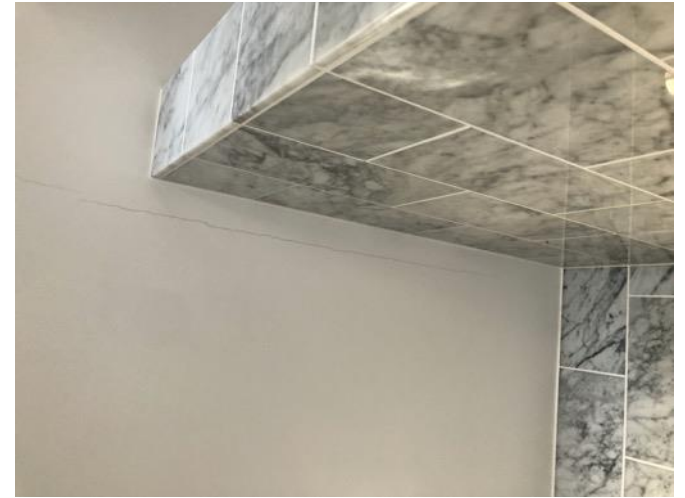
Hairline crack to ceiling
