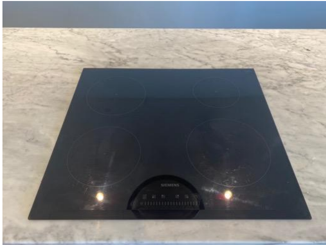
Condition of kitchen hob
