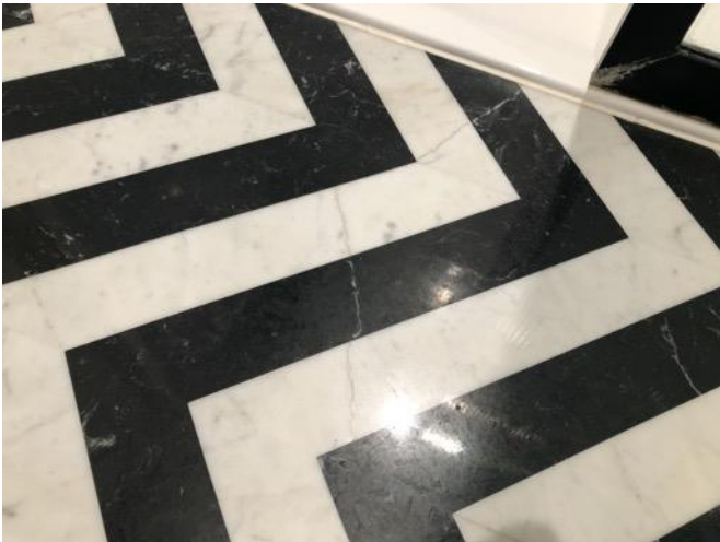
Hairline cracking to floor 3
