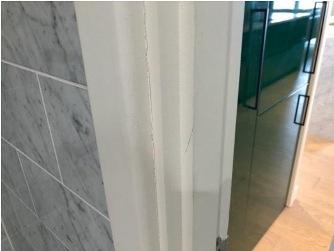
Hairline cracking to door frame
