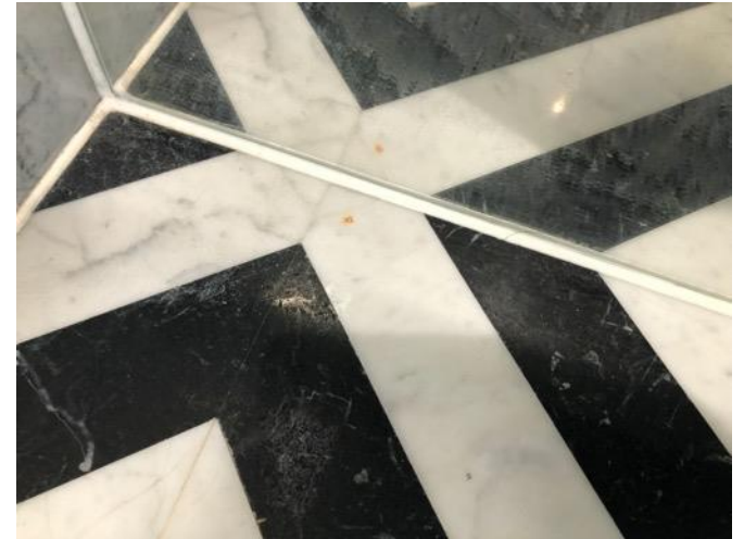
Rust spot mark to floor below hand basin
