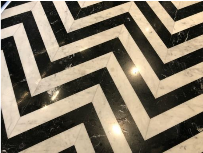
Hairline cracking to floor 1
