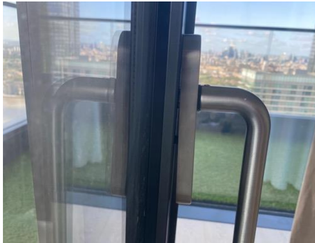
Balcony door handle coming loose from bottom fitting
