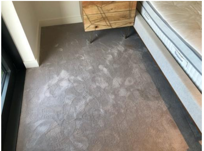
Condition of carpet 2
