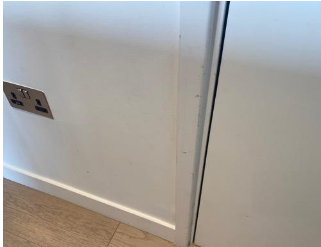
Scuffs/chips to interior front door frame
