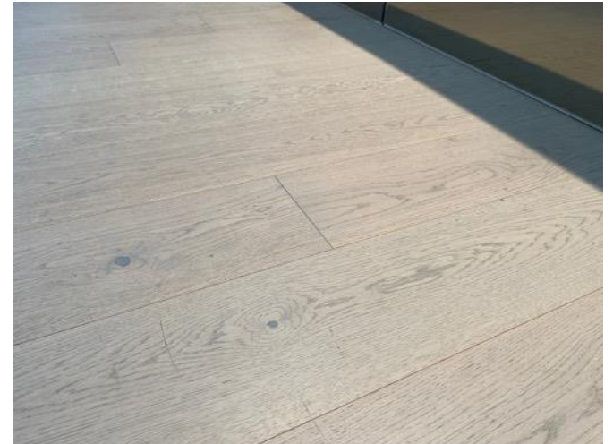
Light scuffs to floor
