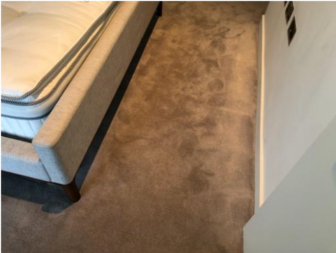
Condition of carpet 3
