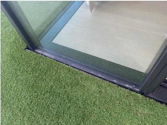
Excess dirt build-up to bottom of window frame
