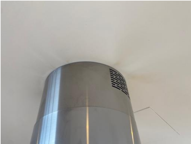
Light shading to ceiling around extractor chimney
