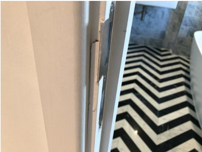
Crack to door frame around lock fitting
