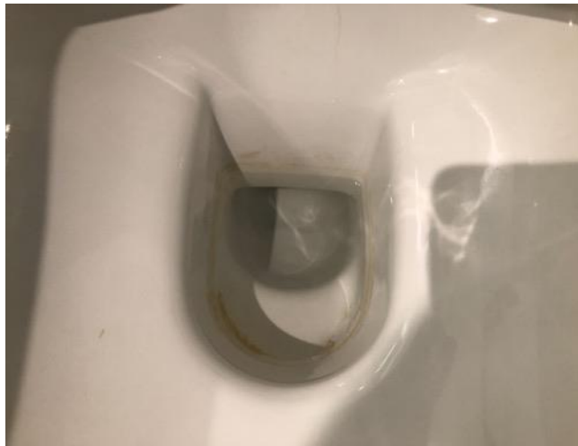
Staining to toilet bowl
