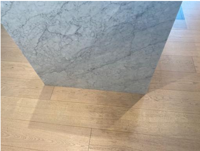
Discoloured patch in front of island area upon entry
