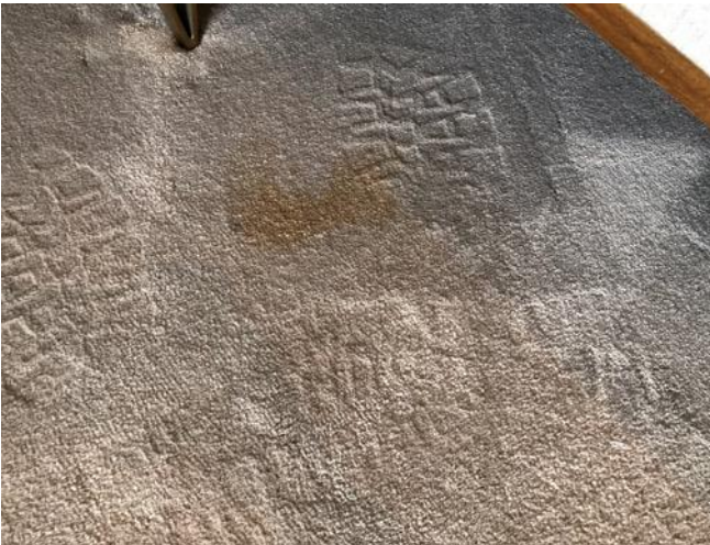
Brown staining to carpet around lhs bedside table 2
