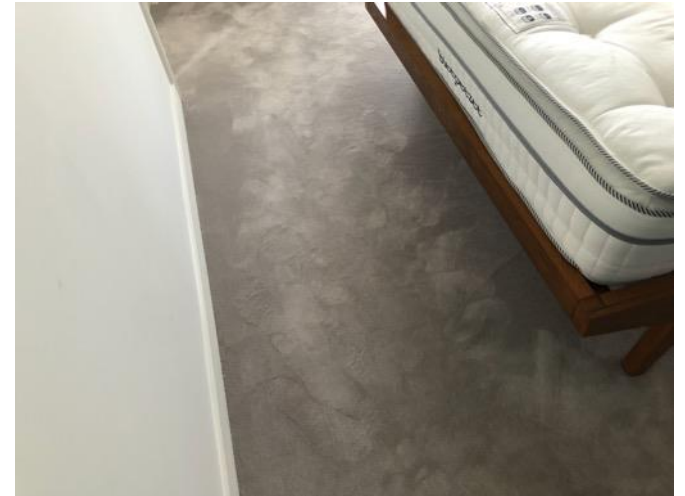
Condition of carpet 2
