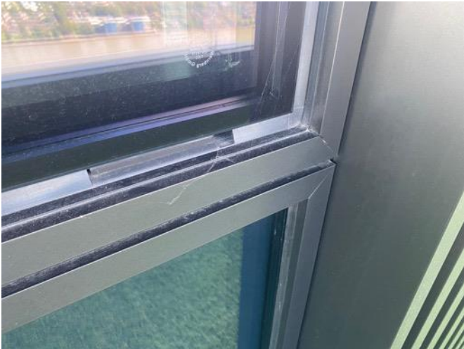
Damage to exterior window frames 2
