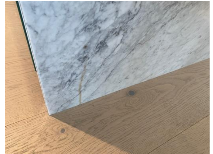
Discoloured mark to island panel facing dining area
