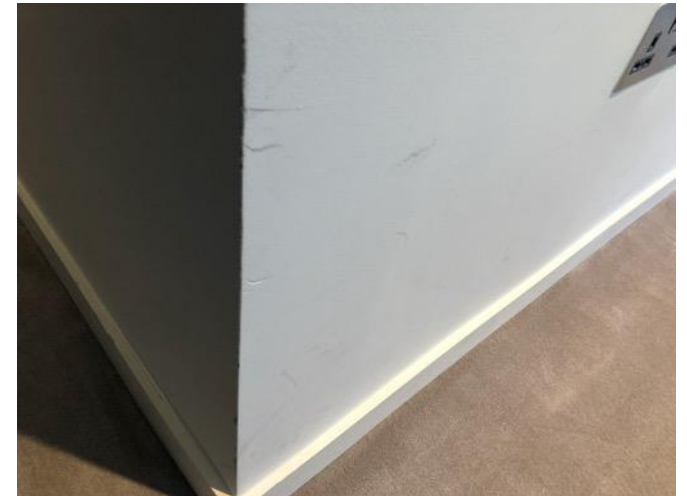
Scuff marks/angle chips to wall
